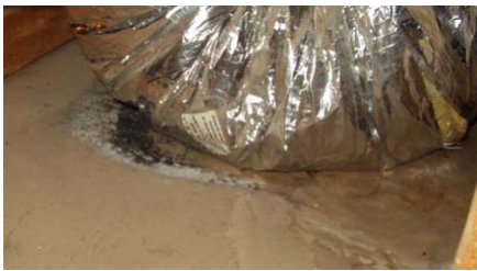
Stachybotrus c. growing in the attic of a Phoenix area home.
